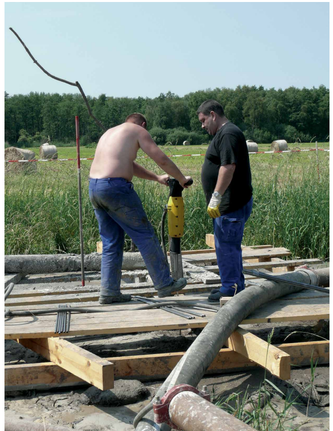
Introduction of the ram injection lances with the ram hammer (photos: Desoi)
